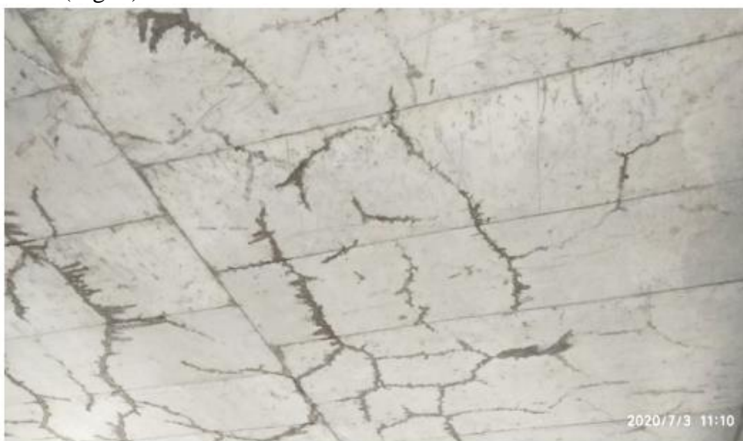
Fig.1. A fragment of the damaged part of a monolithic slab of reinforced concrete beam floor.
