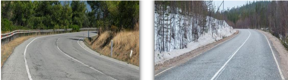
Figure 1. Condition of the road under the influence of the temperature.
