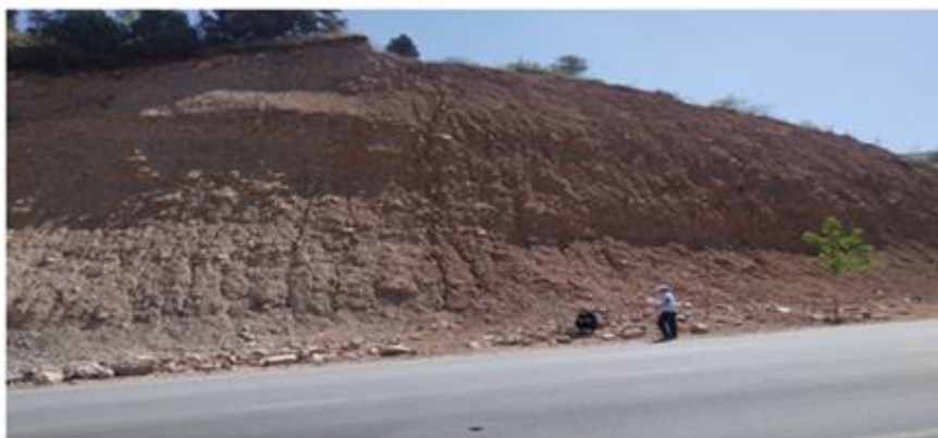
Figure 6. A slope where there is a risk of debris fall
