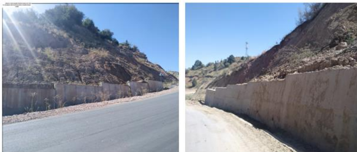
Figure 4. The protection wall was filled with sliding rocks and surpassed some parts
